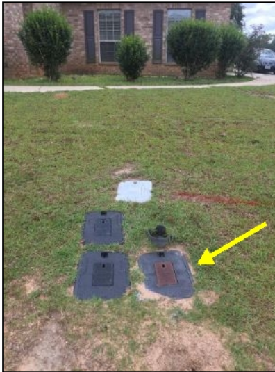
Main Water Shutoff Valve
