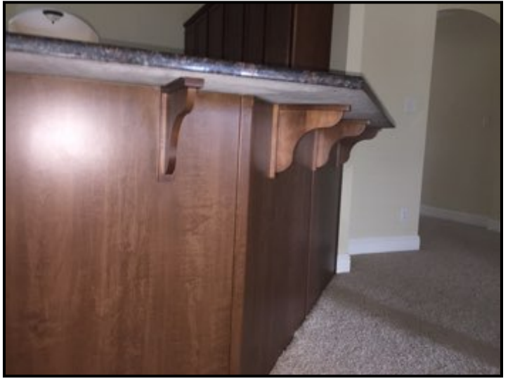
No supports at counter top join.
