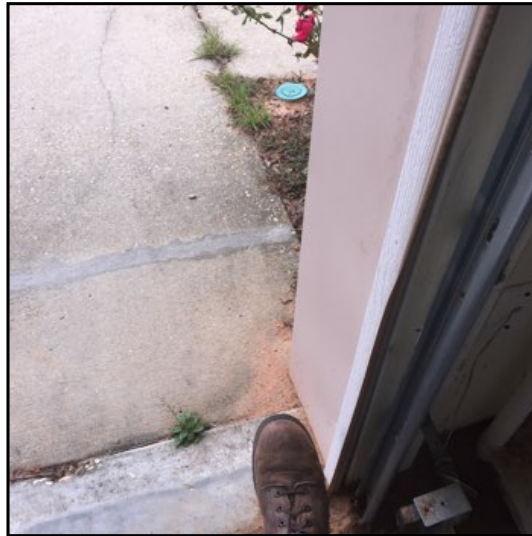
Electric beam functional at time of inspection.
