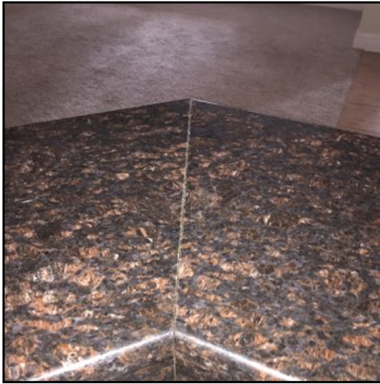
Slight separation of top sections.
