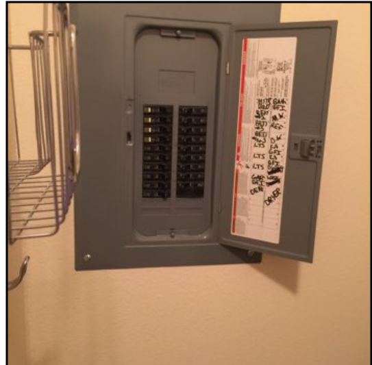
Sub panel located in utility room. Recommend qualified person identify breakers and update general label names.
