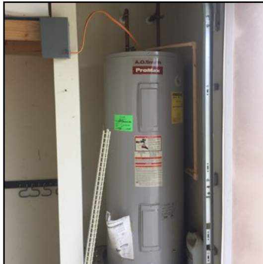
New hot water heater.
