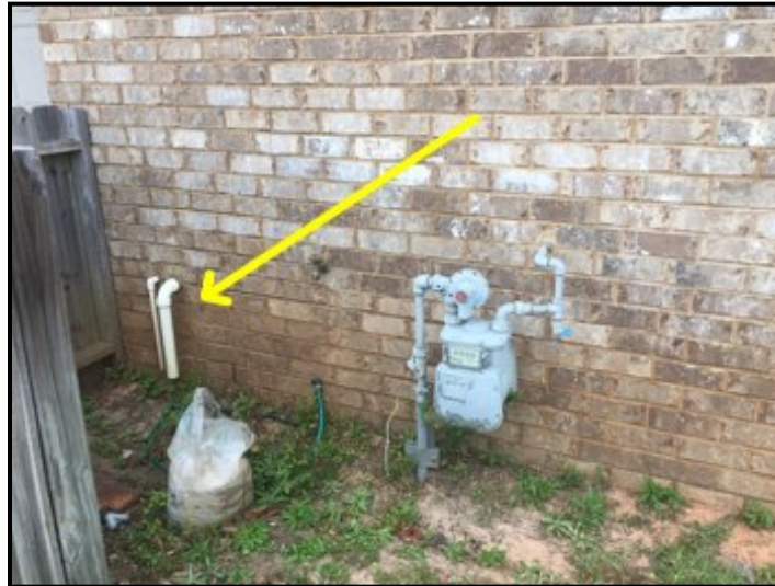
TPRV plumbed to exterior.
