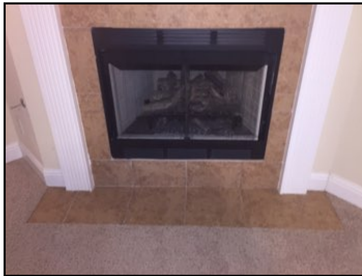
Gas fireplace- functional at time of inspection.
